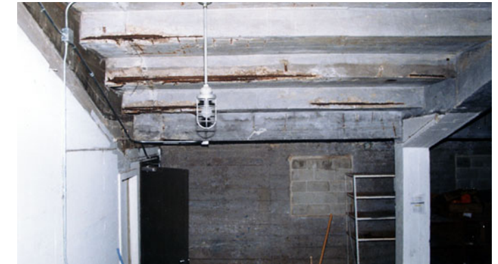
FIGURE 67: Typical interior incandescent fixture. (2002)
