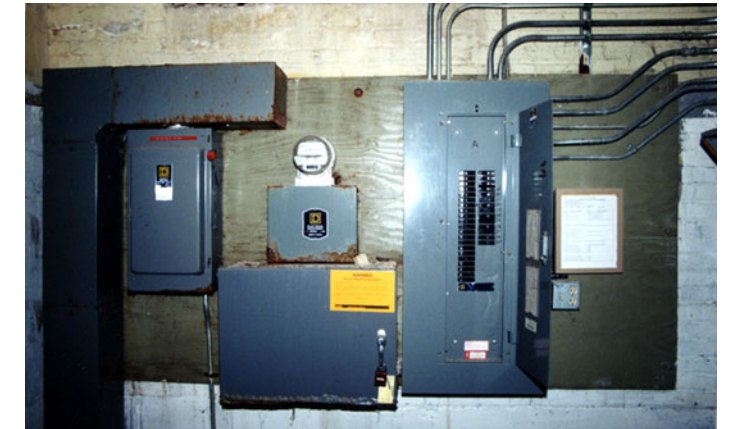
FIGURE 62: Electrical service 'A' (2002)
