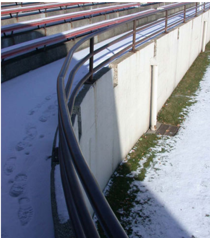
FIGURE 40: Low field wall with drainage scupper and leaders to subsurface drainage system. (2002)
