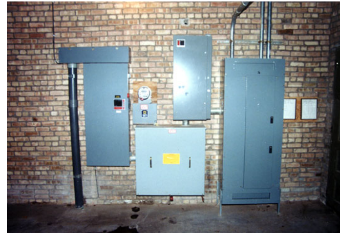
FIGURE 65: Electrical service 'D'. (2002)
