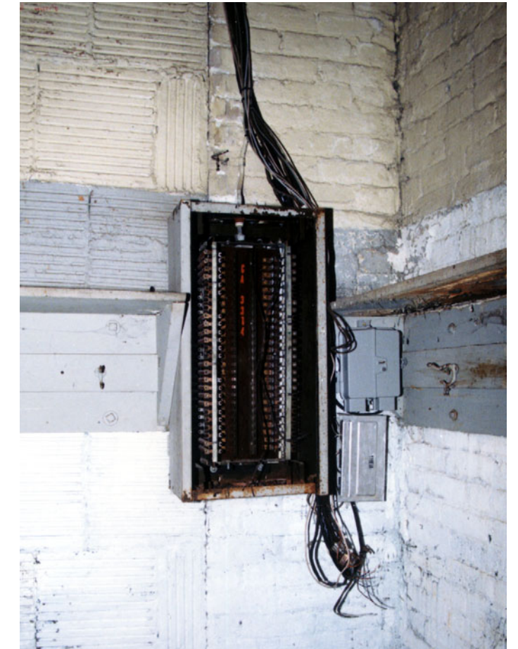
FIGURE 72: Unused and deteriorated electrical equipment to be removed. (2002)
