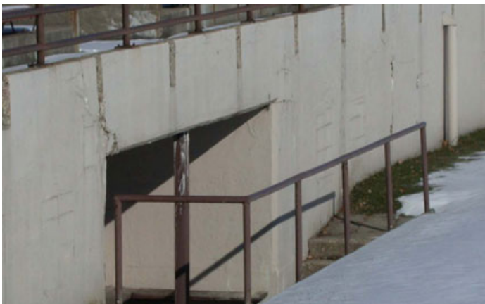
FIGURE 11: Wall damaged from settlement and freeze/thaw cycle. (2002)
