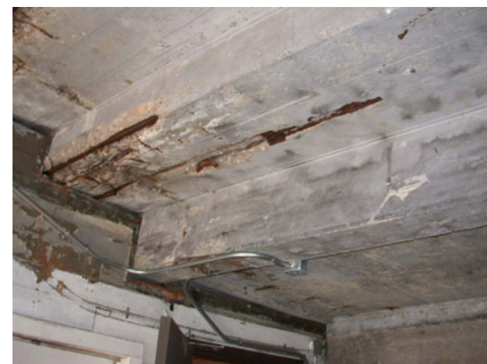
FIGURE 17: Damage to concrete riser slab from water infiltration. (2002)
