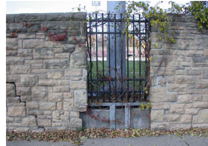
FIGURE 2: Step cracking in the low wall along East Washington Street. (2002)
