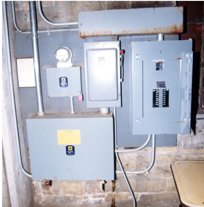
FIGURE 63: Electrical service 'C'. (2002)
