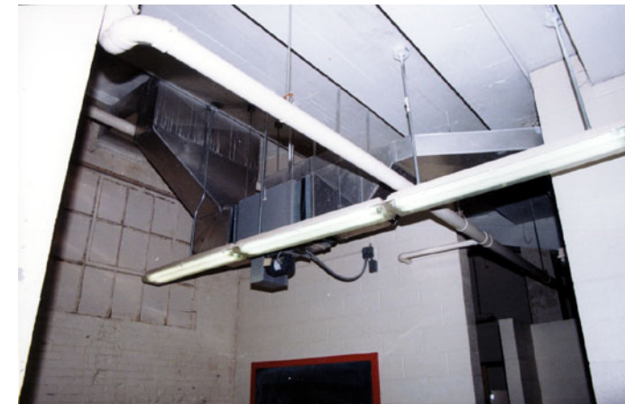
FIGURE 50: Locker room exhaust fan. (2002)
