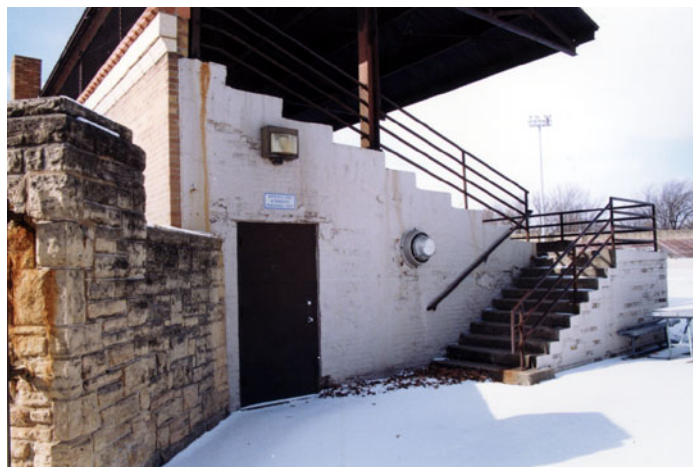
FIGURE 53: Exhaust vent located on the exterior of the building. (2002)
