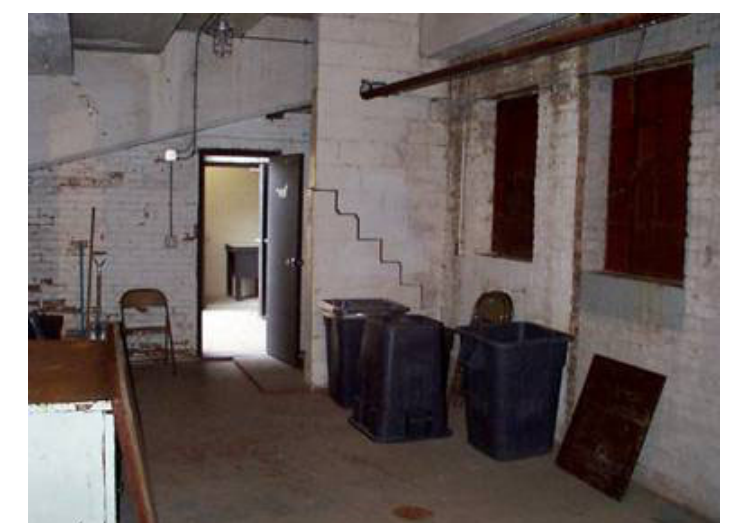
FIGURE 34: Step crack in wall at west ticket booth. (2002)
