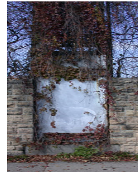
FIGURE 3: Wall opening at one of the light towers along East Washington Street. (2002)
