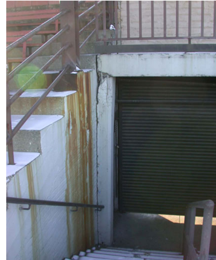
FIGURE 29: Damage to concrete from water infiltration at joints. (2002)
