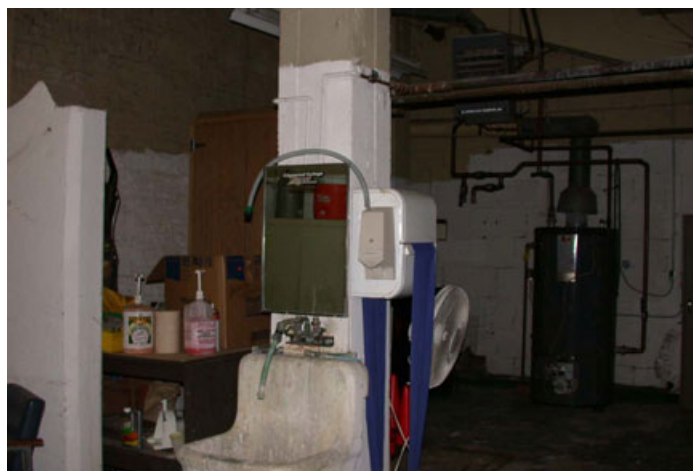
FIGURE 24: View into maintenance room showing utility sink and water heater. (2002)
