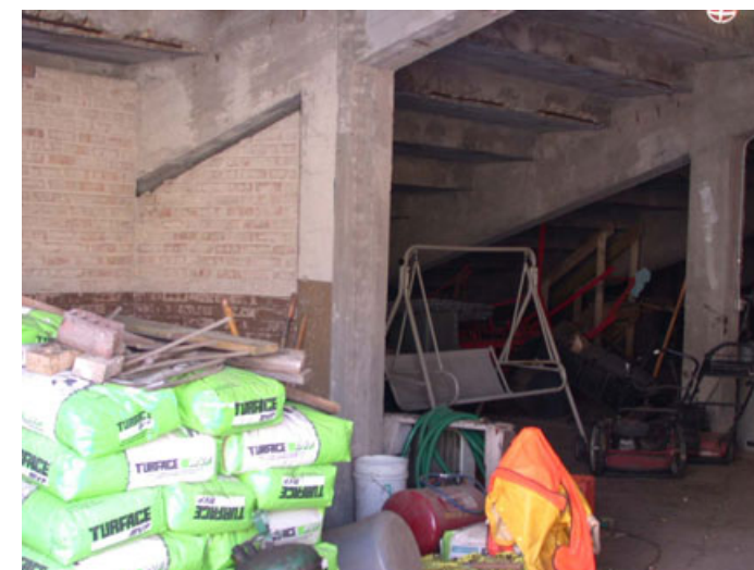
FIGURE 48: Interior of maintenance storage area showing damaged concrete slab. (2002)
