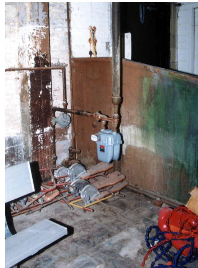
FIGURE 54: Gas meter and regulator inside building. (2002)
