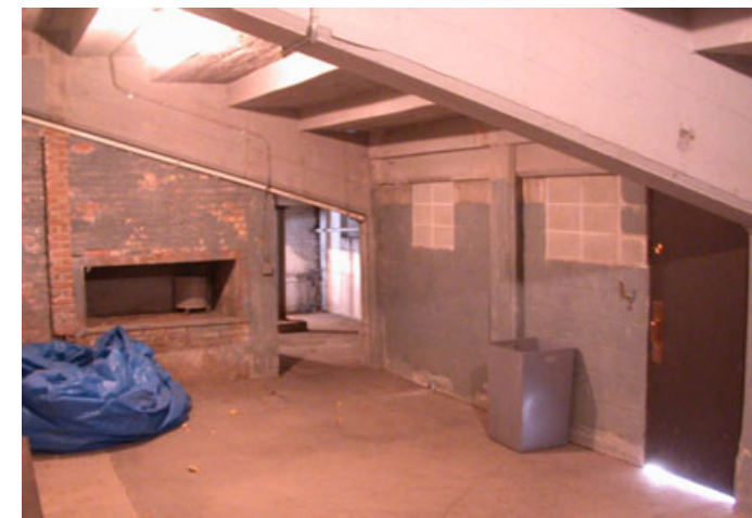
FIGURE 39: Dropped floor level area at base of the stair to the field. (2002)
