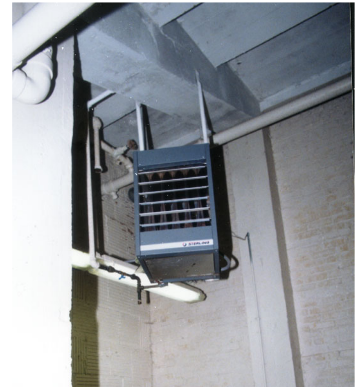
FIGURE 51: Locker room unit heater. (2002)
