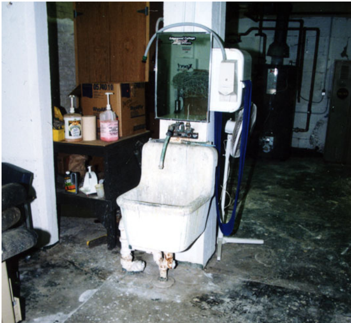
FIGURE 60: Service sink in Maintenance Room. (2002)
