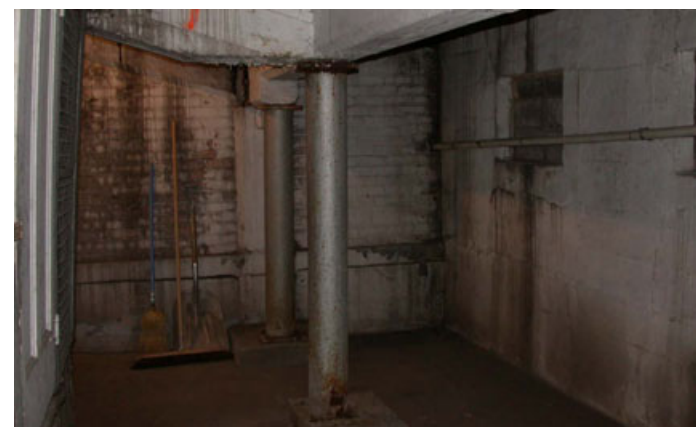
FIGURE 41: Area at base of ramp. Note in-filled windows on wall at right. (2002)
