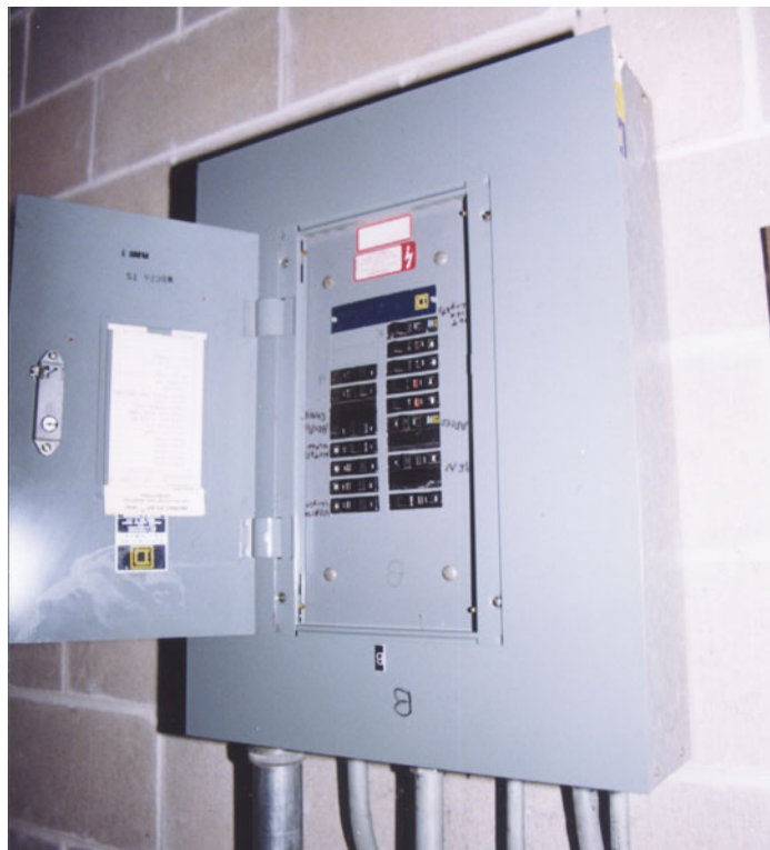
FIGURE 64: Electrical panel 'B' (2002)
