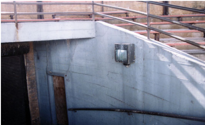
FIGURE 69: Flood light at exit stairs (2002)
