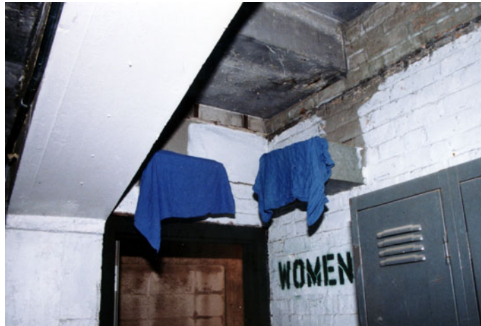
FIGURE 52: Partially dismantled ductwork in the Women's rest room. (2002)
