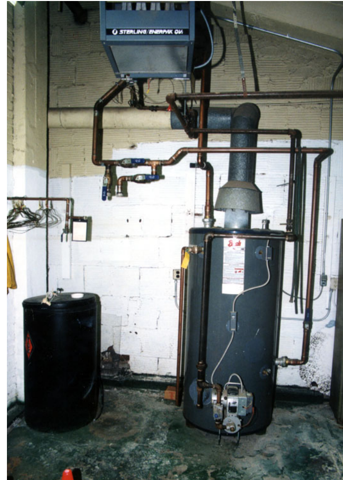
FIGURE 61: Gas fired water heater in Maintenance Room. (2002)
